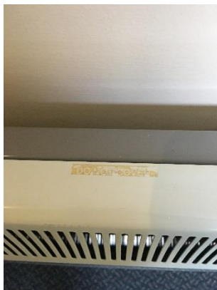
Warning signage has faded
