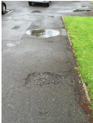
Uneven paths and moss build up leading to potential trip and slip hazards
