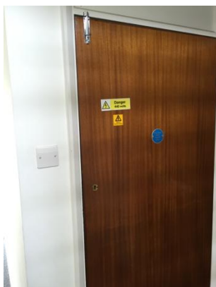
Electrical cupboard doors to be kept locked at all times
